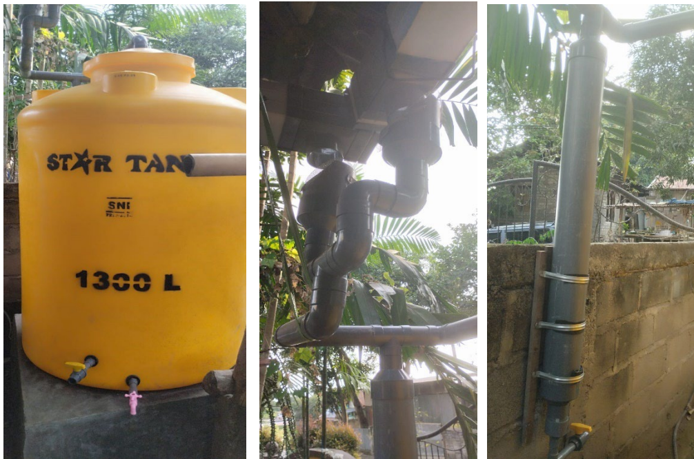
Figure 1. Rainwater Harvesting System
