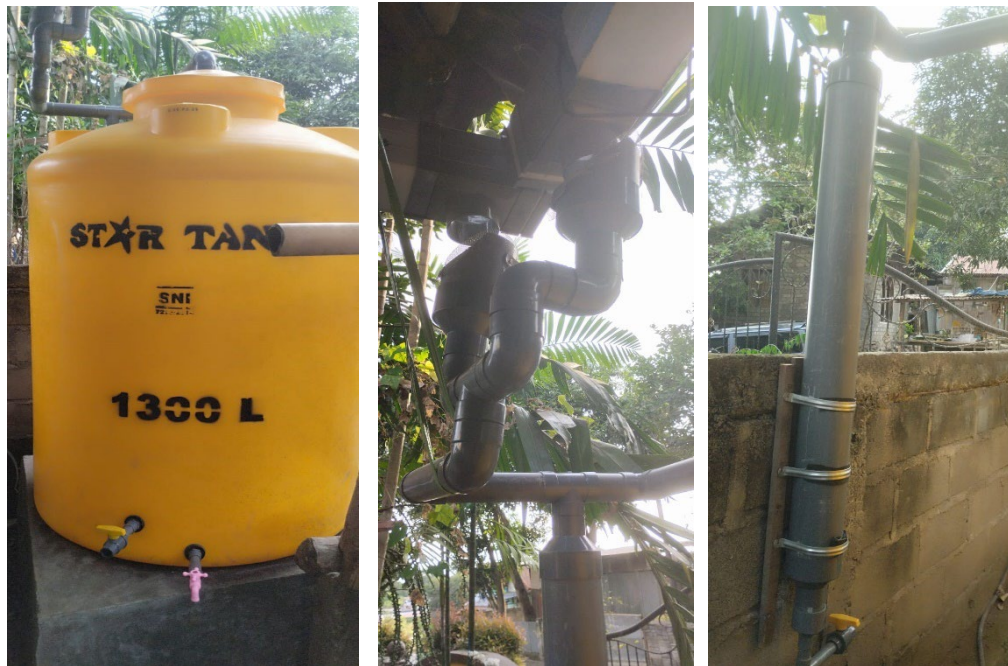
Figure 1. Rainwater Harvesting System
