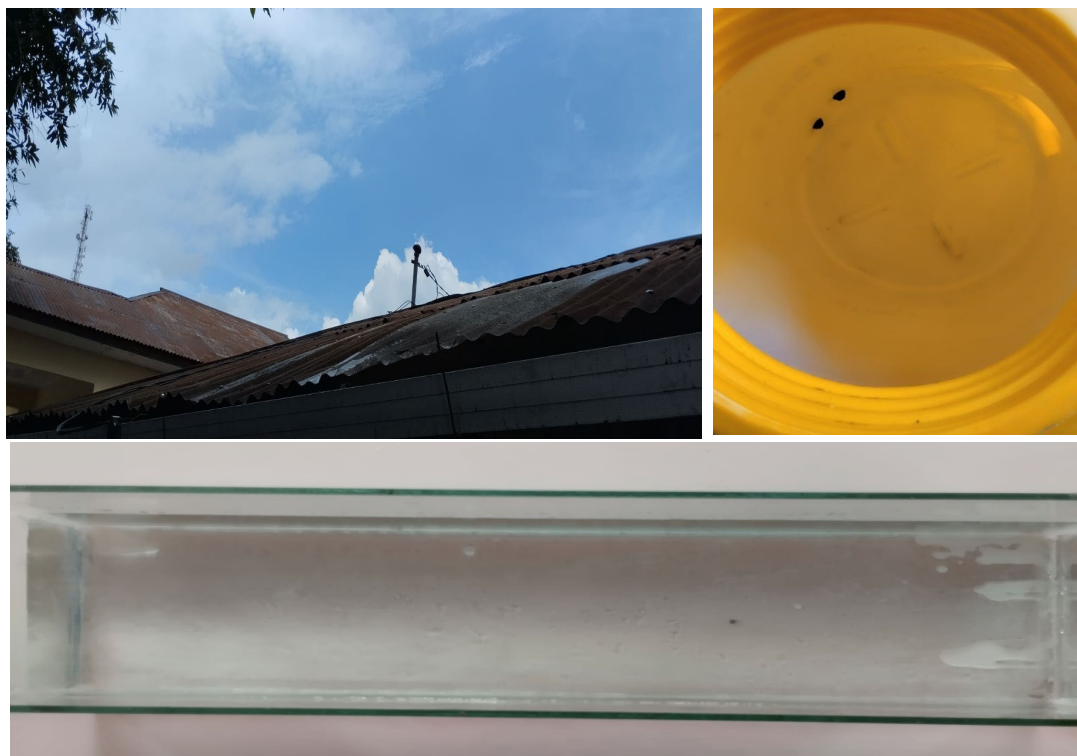
Figure 4. Condition of the roof, the storage tank after cleaning, and the condition of the water inside the storage tank
