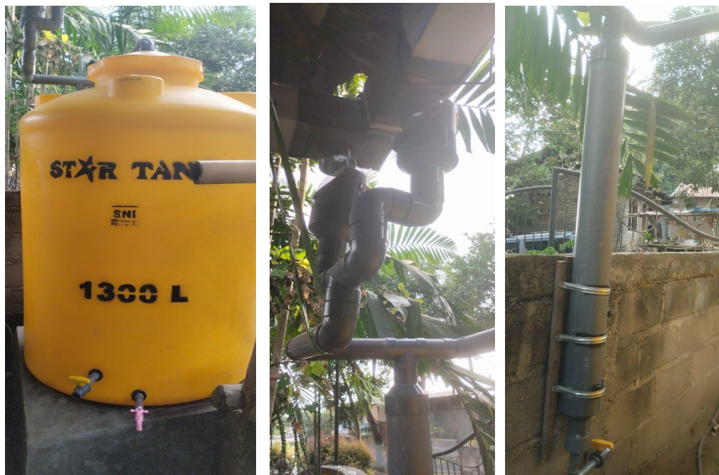
Figure 1. Rainwater Harvesting System
